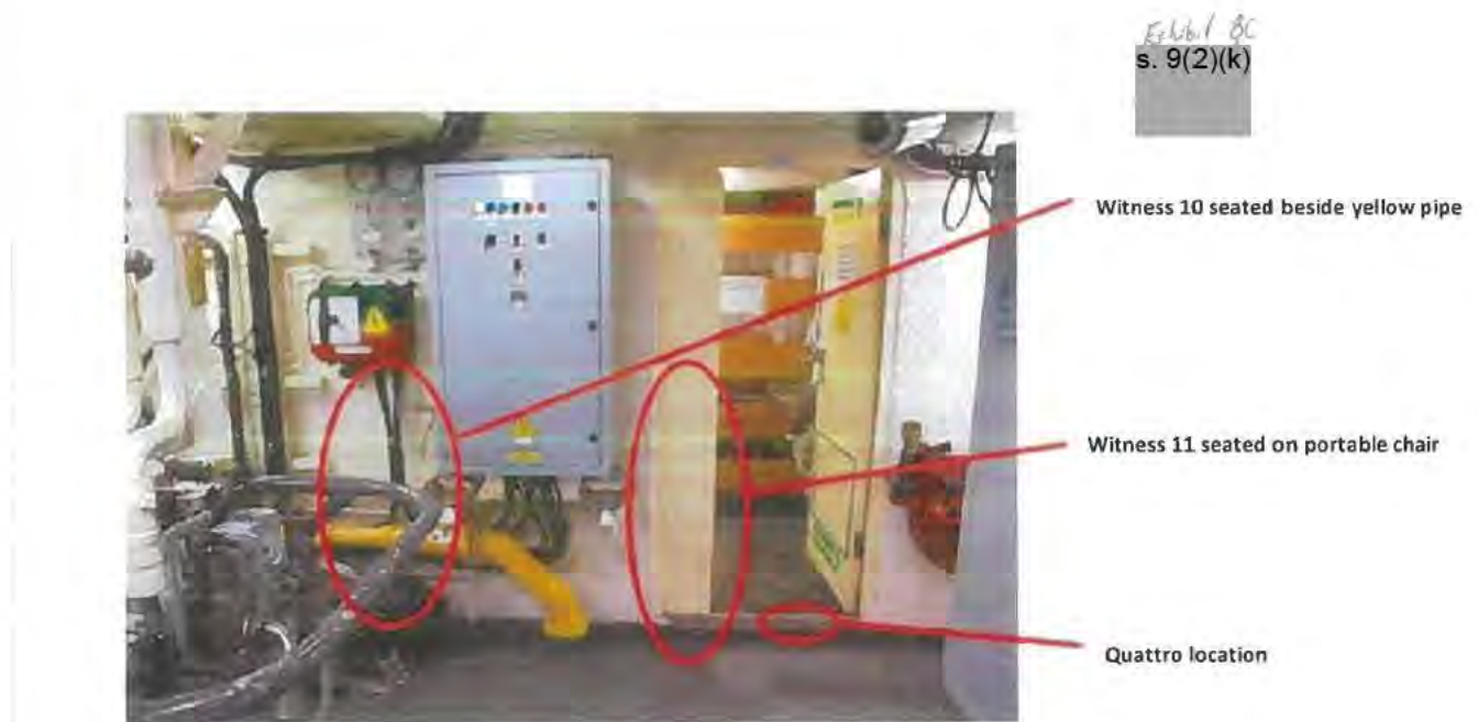
Figure 2 – Location of Witnesses 10 and 11 in Compartment 3M
