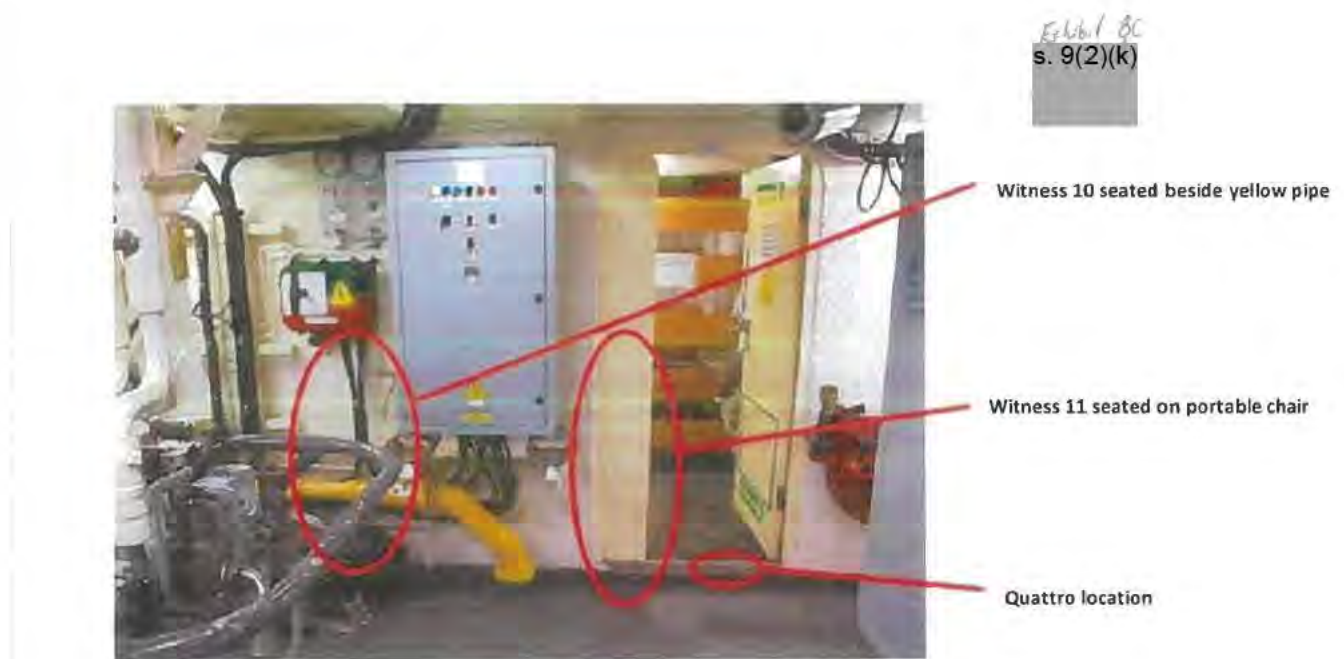
Figure 2 – Location of Witnesses 10 and 11 in Compartment 3M
