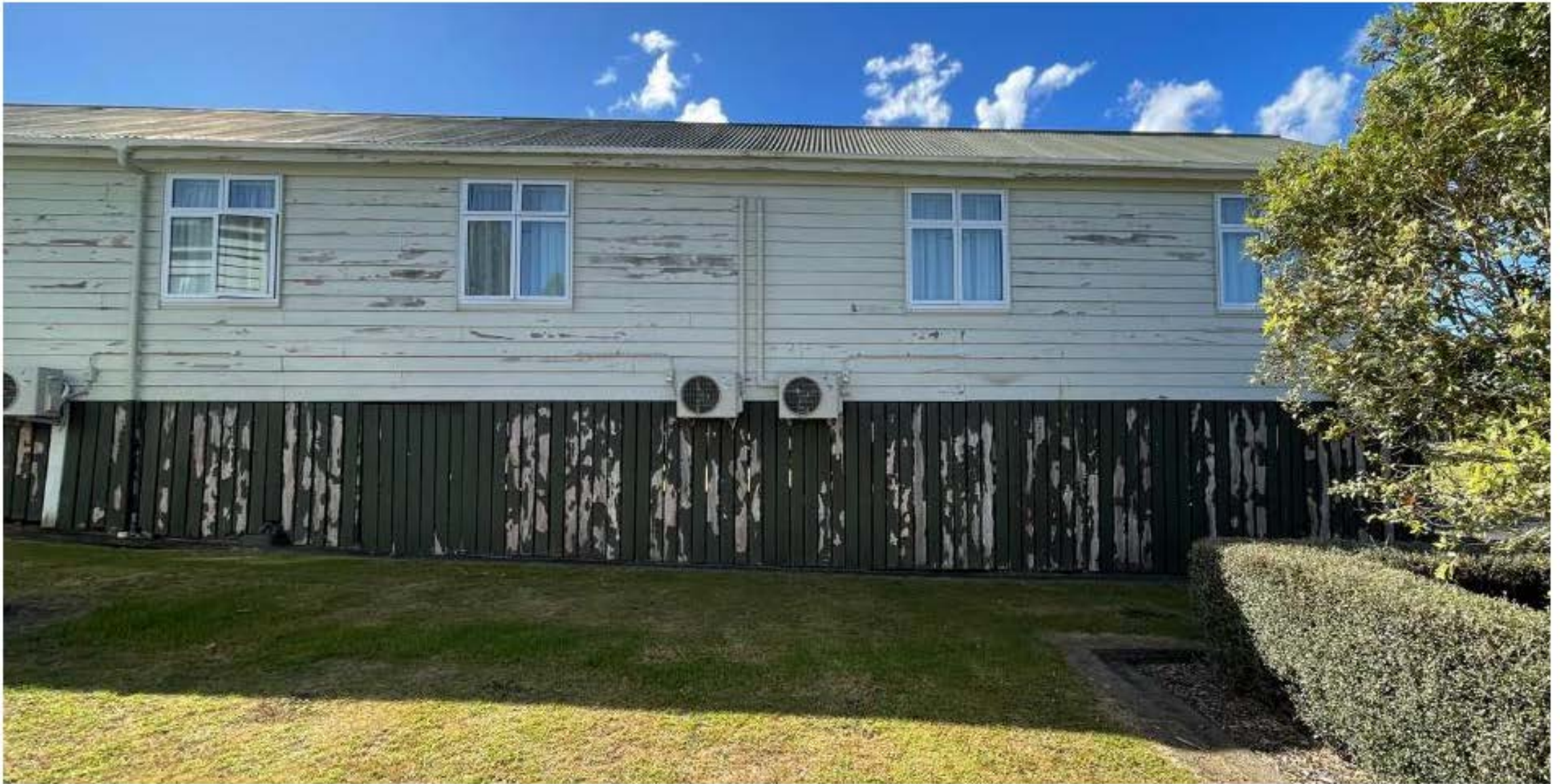
Deteriorating Cladding of Hume Block
